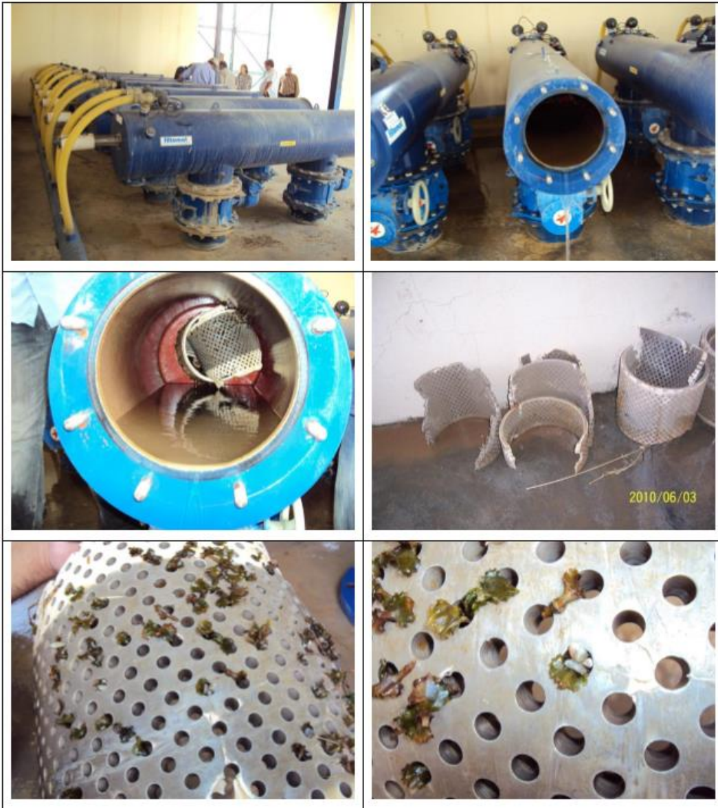
Figure 13 .Urfa Bozova Irrigation Pump Station's Filters in 2010 (21)
