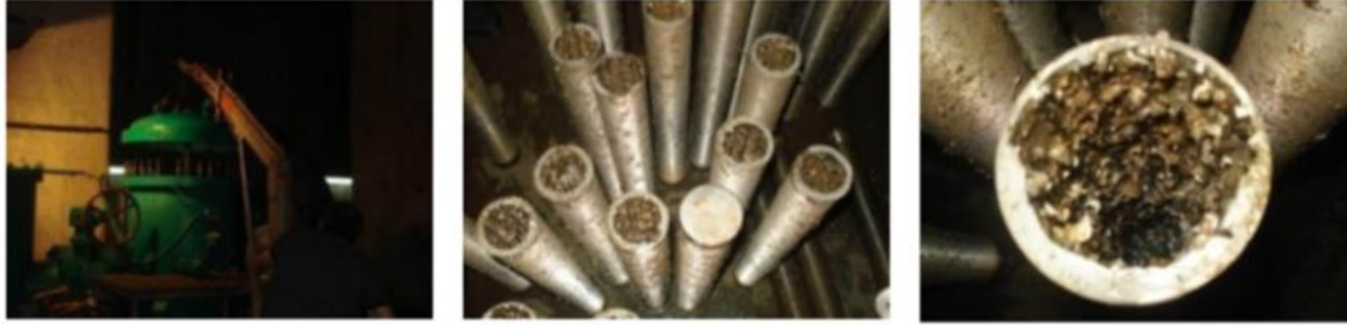
ATATÜRK Dam HEPP Cooling system
