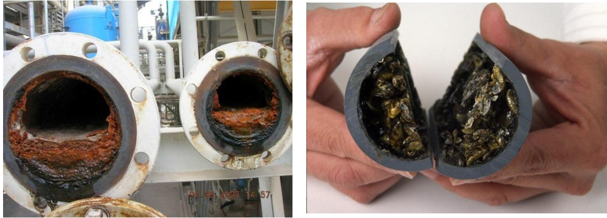
Figure 16. Zebra Mussel accumulation in the pipes.
