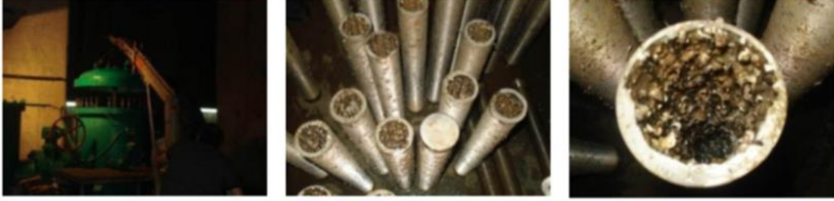
ATATÜRK Dam HEPP Cooling system
