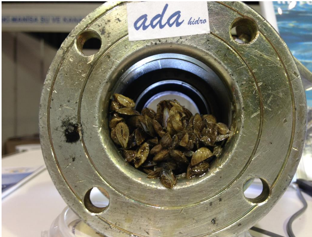
Figure 9. Zebra Mussel accumulation in a pipeline
